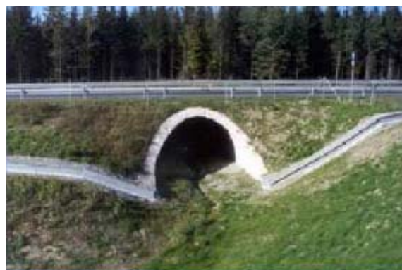
Figure 4.6: Arch culvert with fence for large mammals and lipped wall for amphibians (FHWA/US DOT 2002)
