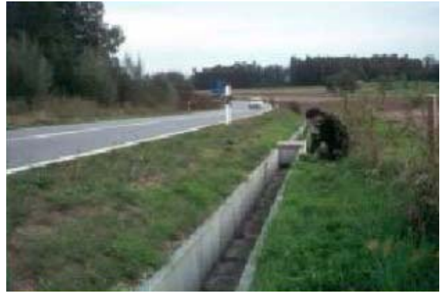
Figure 6.5: Concrete trench and drop inlet with one-way pipe for amphibian crossing (FHWA/US DOT, 2002)
