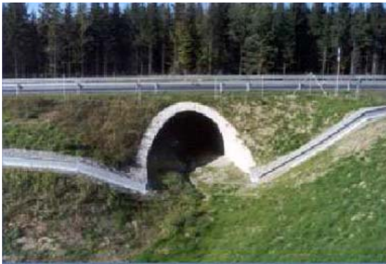
Figure 6.10: Arch culvert with fence for large mammals and lipped wall for amphibians (FHWA/US DOT, 2002)
