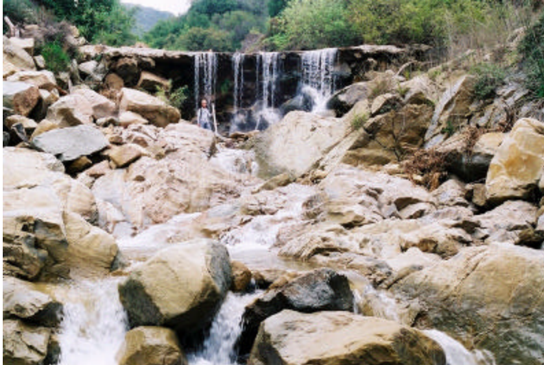
BR_RN_13: Failed Road Crossing
