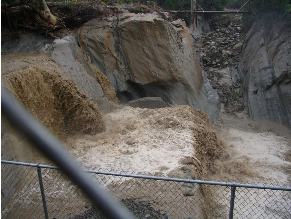
Damage to dam during 2005 flood
