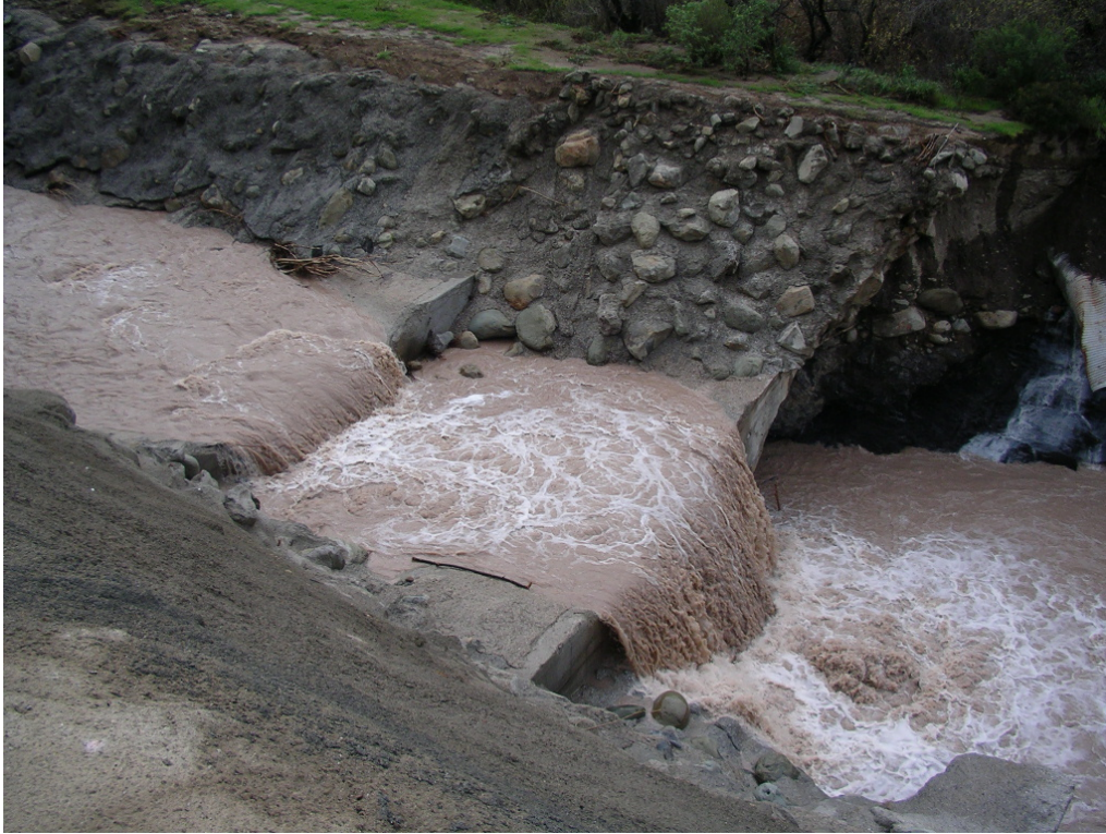
Failure of downstream grade controls following 2005 flood
