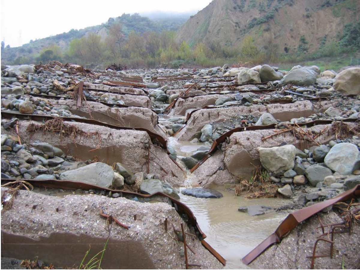
Fishway failure following January 2005 flows
