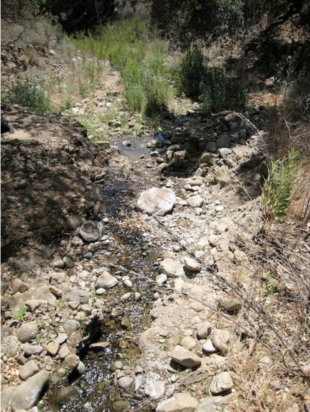
Looking downstream from the top of the incising channel.
